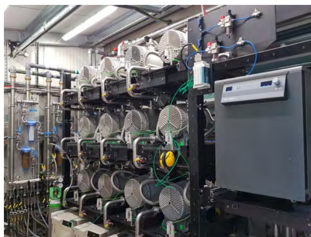
Figure 5: Pumps and compressors are now housed in a separate plant room that opens out onto the back of the building. By segregating these from the experimental stations, we achieve major improvements in noise, and we free up space in the lab.
