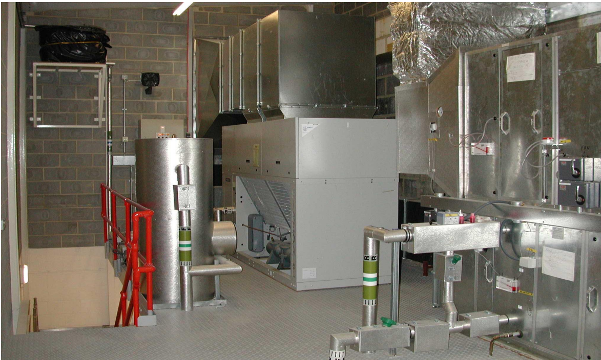
Photo 5. Air Conditioning Plant on 1 st Floor of new Plant Room.
