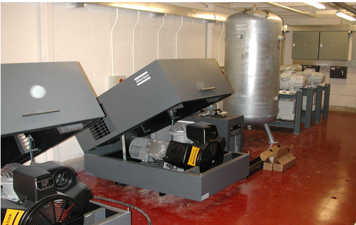
Photo 6. Vacuum pumpsets and Let up compressors and receiver on Ground Floor of new Plant Room.
