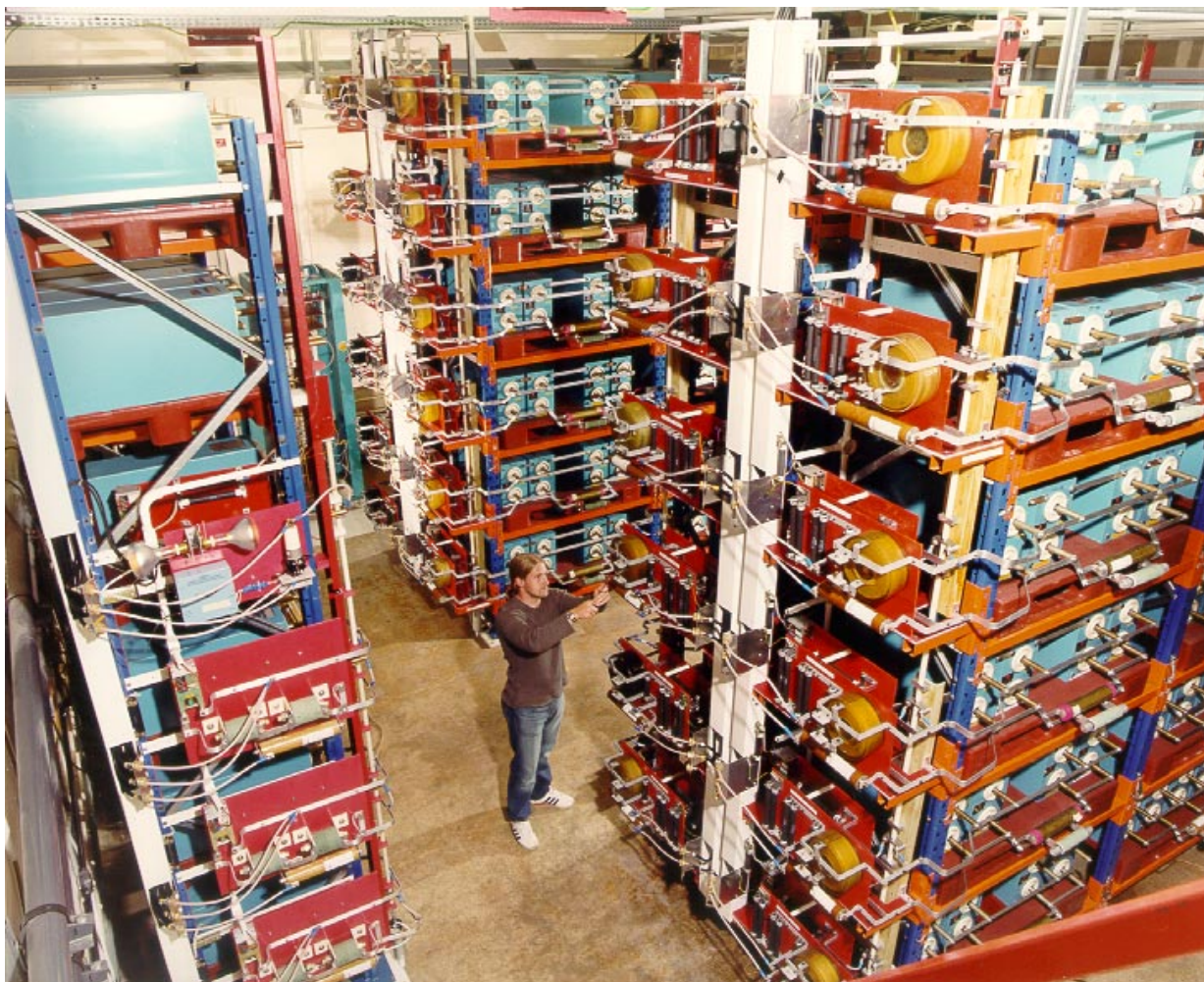
Figure 1. Paul Holligan of the CLF Electrical Engineering Section adjusting a PFN following installation of the new Vulcan pulsed power area.
